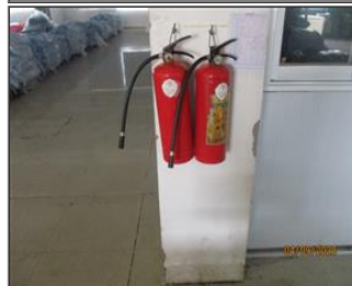
Photo of fire safety equipment Fire extinguishers.JPG
