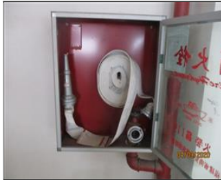
Photo of fire safety equipment Fire hydrant.JPG
